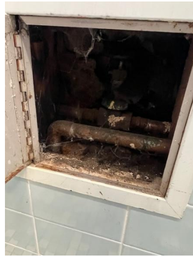
Plumbing access in girls RR
