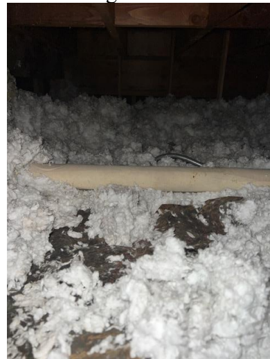
attic pipe insulation
