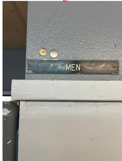
Hall sheet rock wall material
