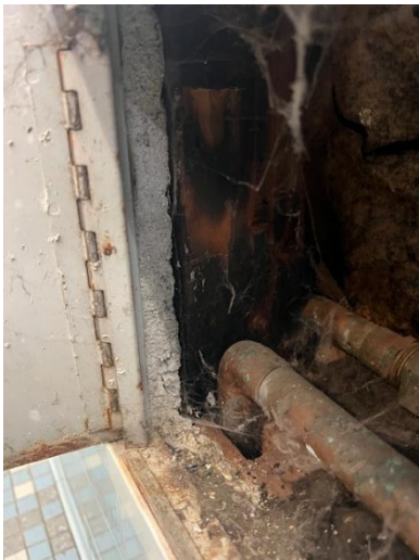
Plumbing access in girls RR
