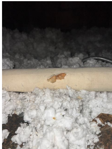
attic Pipe Insulation
